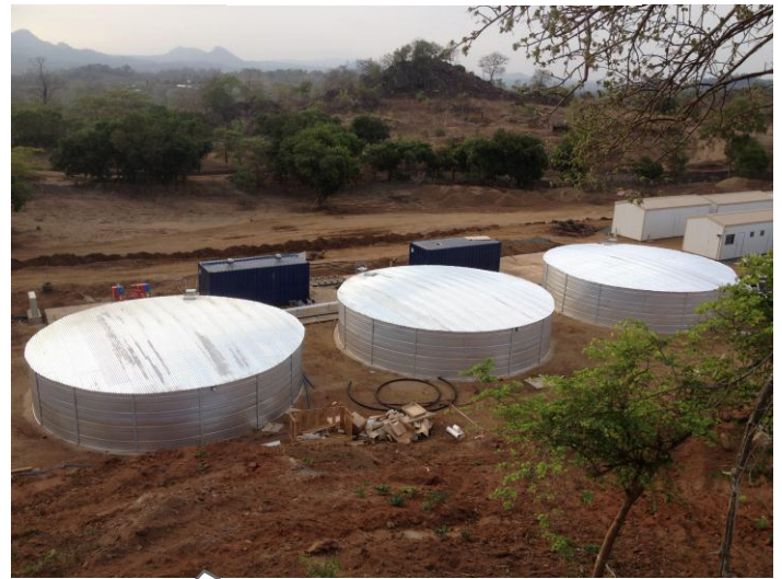
Typical design of 2 x 15m 3 /hr containerized potable water treatment plant & 2 x 2.7m 3 /day RO processed water for Nacala Corridor Project in Malawi as phase 1 at two sites. Modular and at marginal cost increase production by 100%
