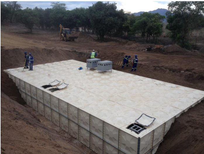
Typical design of 2 x 400 people sewerage plant for Nacala Corridor Project in Malawi as phase 1 at two sites. System is modular and will be increased as the people requirement for this camp increases.
